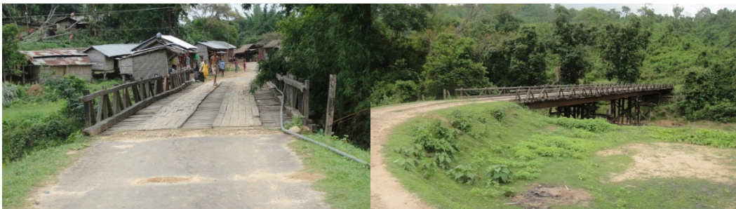
Two of the many Semi Permanent Timber Bridges (SPT) in the State. These are vulnerable to flash floods & require regular repair and decking replacement. Many of these have been replaced by RCC bridges in the 11 th Plan, many more remain
